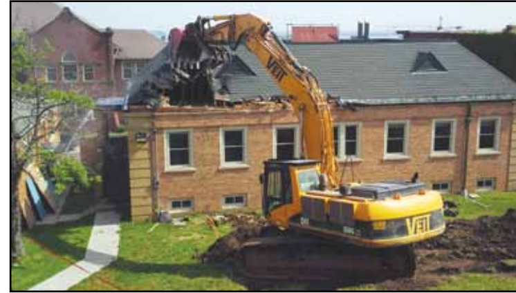
The old CAIR building being torn down to make room for the new CAIR facility to help bring health services to Band members and other eligible people.
