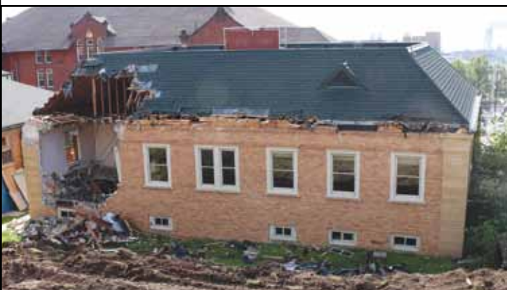
The hole on the backside of the CAIR facility just shortly after deconstruction began.
